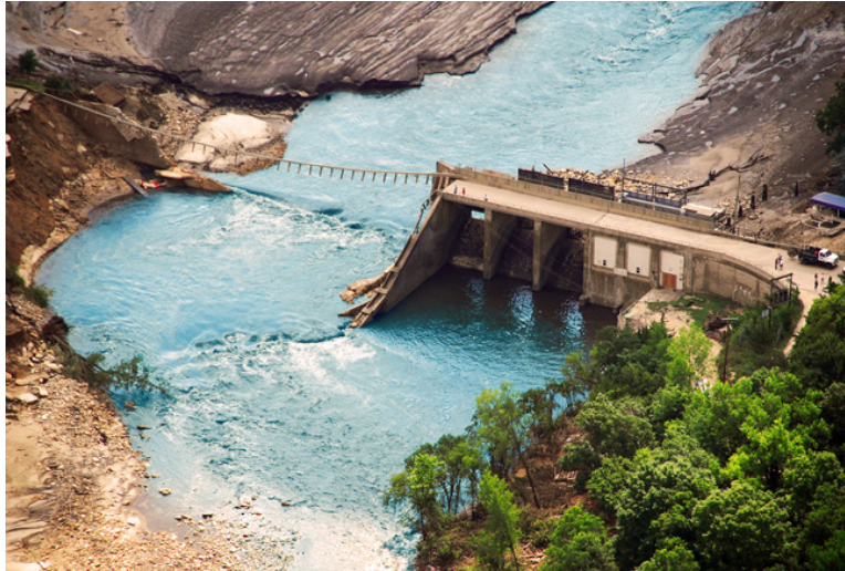
Photo 3. Delhi Dam failure (courtesy of Iowa Wing Civil Air Patrol)
