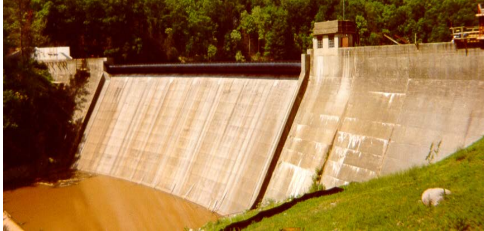
Photo 6. Sugar Hollow Dam: inflatable bladder crest gate
