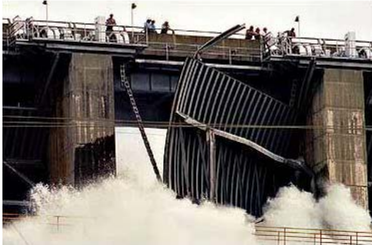
Photo 2. Gate failure at Folsom Dam, 1995 (courtesy of Bureau of Reclamation)
